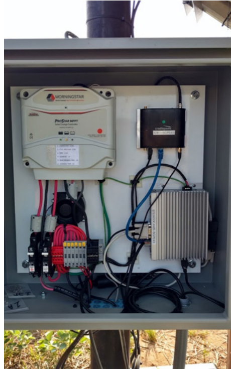
Figure 3. Interior of the electrical enclosure of a camera setup. A charge controller, a cellular modem, a minicomputer, and circuit breakers and fuses are enclosed in this box, placed beneath the solar panels as shown in Figure 2.
