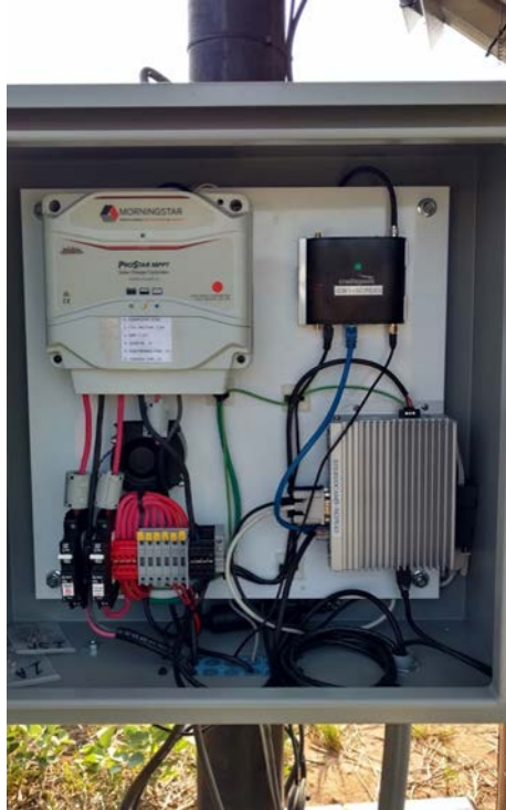
Figure 3. Interior of the electrical enclosure of a camera setup. A charge controller, a cellular modem, a minicomputer, and circuit breakers and fuses are enclosed in this box, placed beneath the solar panels as shown in Figure 2.
