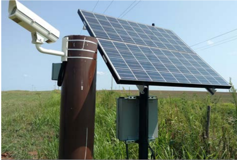
Figure 2. A camera setup onsite. Two solar panels mounted with a top-of-pole rack, an electrical enclosure beneath the solar panels, and the camera enclosure tilted approximately 18° from the ground.
