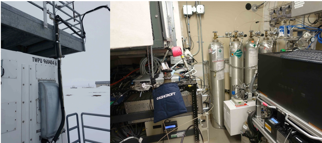
Figure 1. Inlet on NSA shelter (left) and instruments (right) inside NSA shelter. The black insulated inlet extended from the northeast corner of the shelter roof at the level of the handrail. Within the shelter were the LGR CO/OCS/CO 2 /H 2 O instrument (left side of photo) and the Aerodyne 13 CH 4 / 12 CH 4 /C 2 H 6 instrument.
