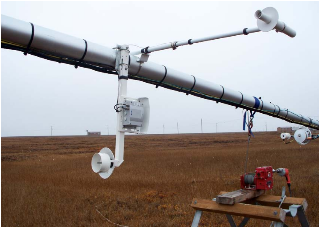
Figure 1. HMT337 Installation at Atqasuk.
