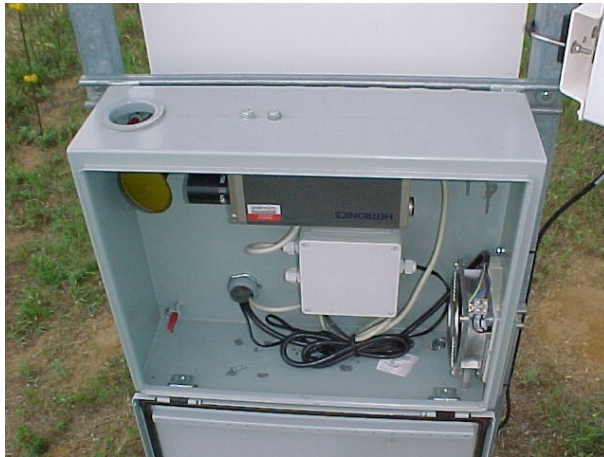
Figure 4. Interior of the infrared thermometer enclosure.
