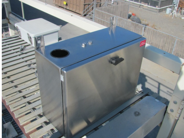
Figure 3. Exterior of the infrared thermometer enclosure.
