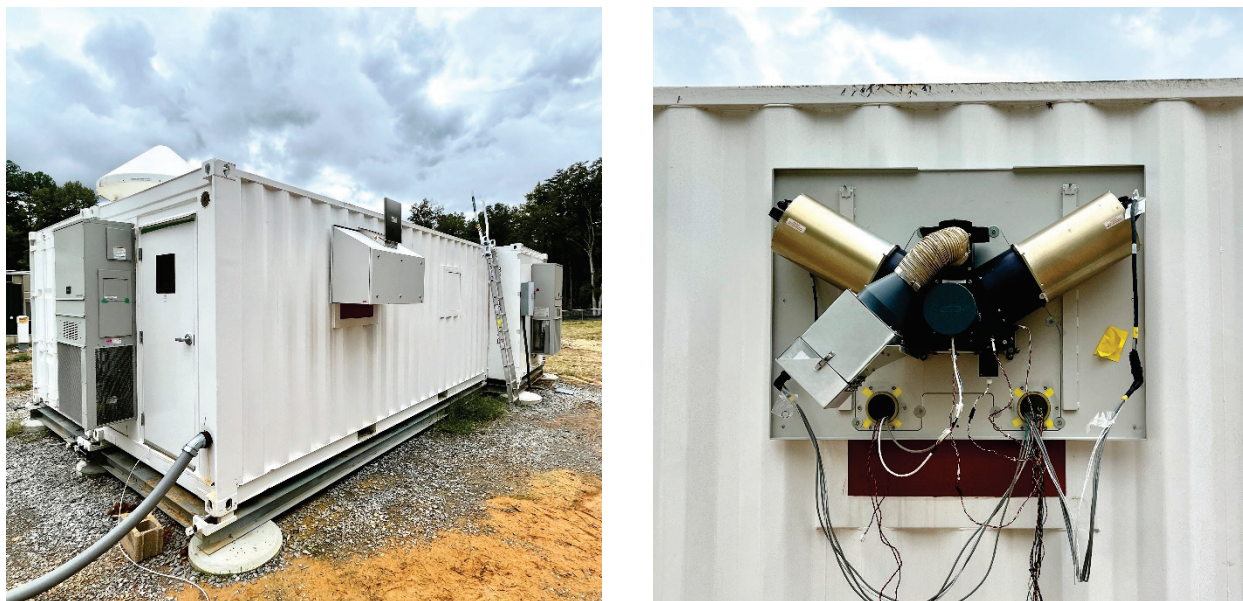
Figure 2. AERI front-end at BNF M1 site (left). Protective enclosure removed, showing blackbodies, sky aperture, and fan (right).
